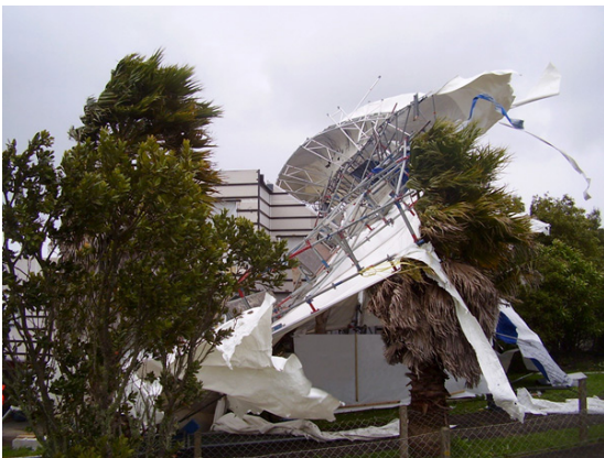
Fig 4: Strong winds tore a sheeted scaffolding system from this building
