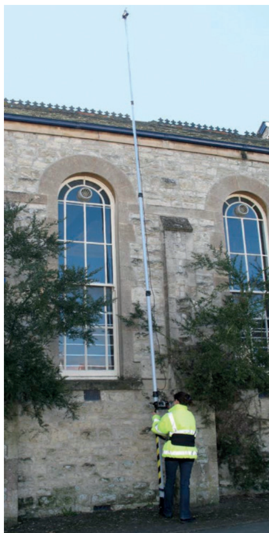
Figure 1: Remote inspection mast with hand-held lightweight CCTV system (Image courtesy of Survey Support Ltd) UK
