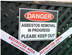
Warning signs must be put up at site entry and all entries into the building
