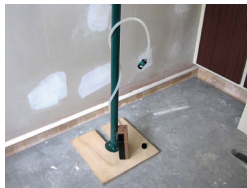
Air must be monitored for asbestos levels outside the enclosure
