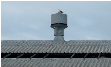
Non-friable asbestos - corrugated roofing
