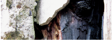
Non-friable asbestos may become friable after being exposed to fire
